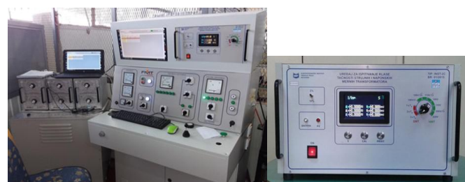
Fig. 14 Automatic device for accuracy testing of 3 current transformers simultaneously [55]
