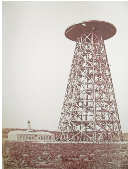
Fig. 5. View of the construction of the tower and auxiliary building of the laboratory, without the dome/electrode that was erected at the very end of the construction (Nikola Tesla Museum heritage).
