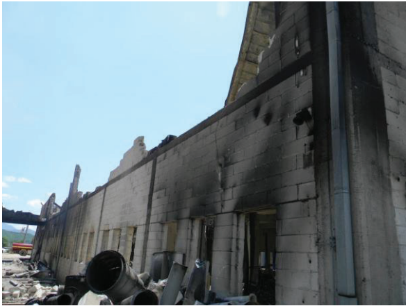
Fig. 3 Damage to the Wall of Hall 2
