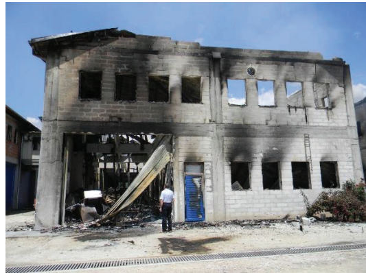
Fig. 2 Main Entrance Appearance to Hall 2 After the Fire
